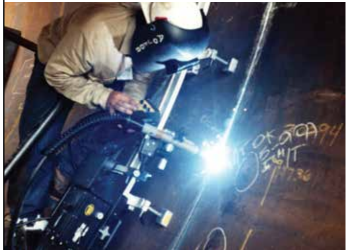
Shown Above - Vertical linear weave welding with ARM-2480 Support Bar w/ Magnets
